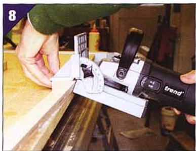
Set the biscuit jointer to cut the slots at 22.5 degree, and cut the matching slots in the leg components
