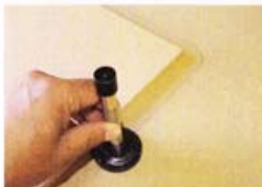
▲ Pic. 3 The result is an accurate template of the area to which the board will be fitted. It's narrower all round by the wheel offset, of course, but this is corrected later
