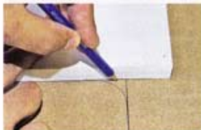
▲ Pic. 4 You'll need to extend the lines where the scribing wheel goes around a corner as it will have been radiused by the wheel
