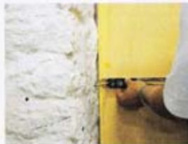
▲ Pic. 2 Using the level to keep it on track, the Multiscribe is worked along the edge to be traced
