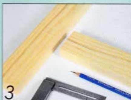
3 Mark the centre of the joint with a sharp pencil and a small square
