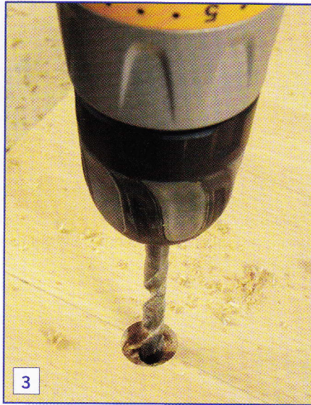
3 Use the centre hole created by the spade bit to centre the drill bit
