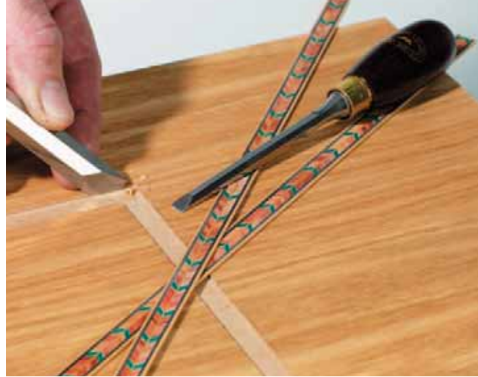
Use a sharp chisel to remove the rounded corner left by the router cutter, taking care not to widen the recess.
