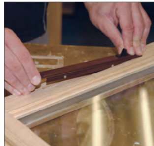
And fit both sides of the Trickle vent. The system produces a 12mm groove for a standard Trickle Vent.
